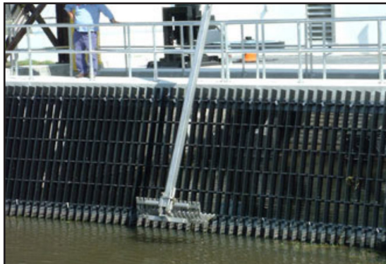
Racks showing corrosion due to impact
